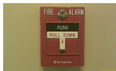
Fire Alarm Station (Three on each floor)
